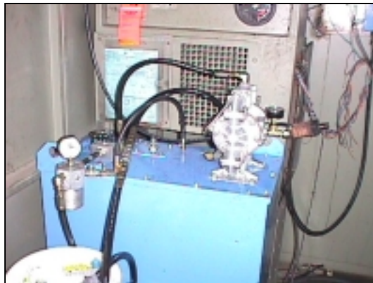
Figure 2: KELTRACK Reservoir Tank & Primary Pump
